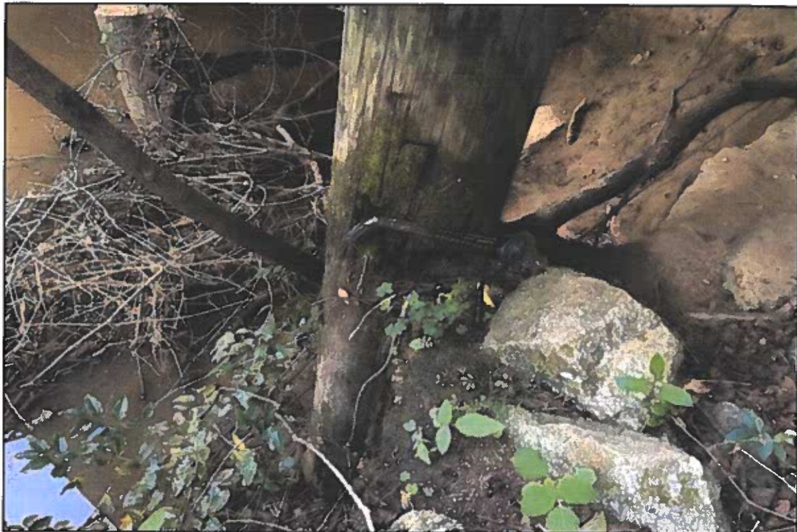
Pile 1, bent 2 is 100% rotten
